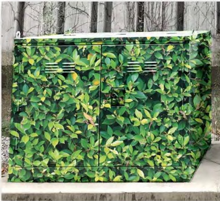
Figure 15: Vinyl Screen Wrap of Transformer
